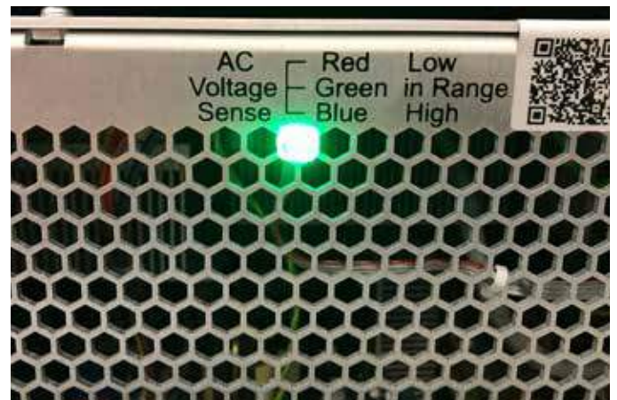
LED indicates facility power is OK.
